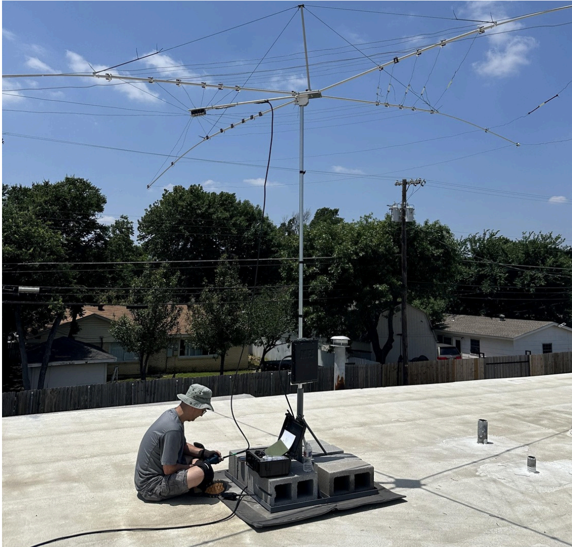
John, KF5PHP working on the cobweb antenna as part of the work party
